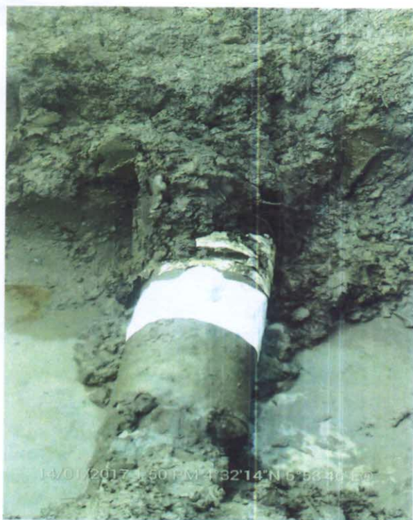
LEAK POINT AFTER REPAIR
